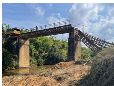
Bridge that collapsed © D. Roullet
